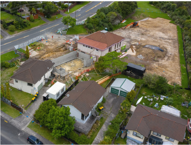
Above: Bishop Ross 'turned the first sod' to launch construction in September 2020; An aerial view of the building site in November 2020.
